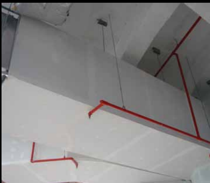
From top: External walls at Kim Chuan Depot, structural steel beam cladding at Chartered Semiconductor of Woodlands and post cladding of steel ducts at ION Orchard. All projects in Singapore.
