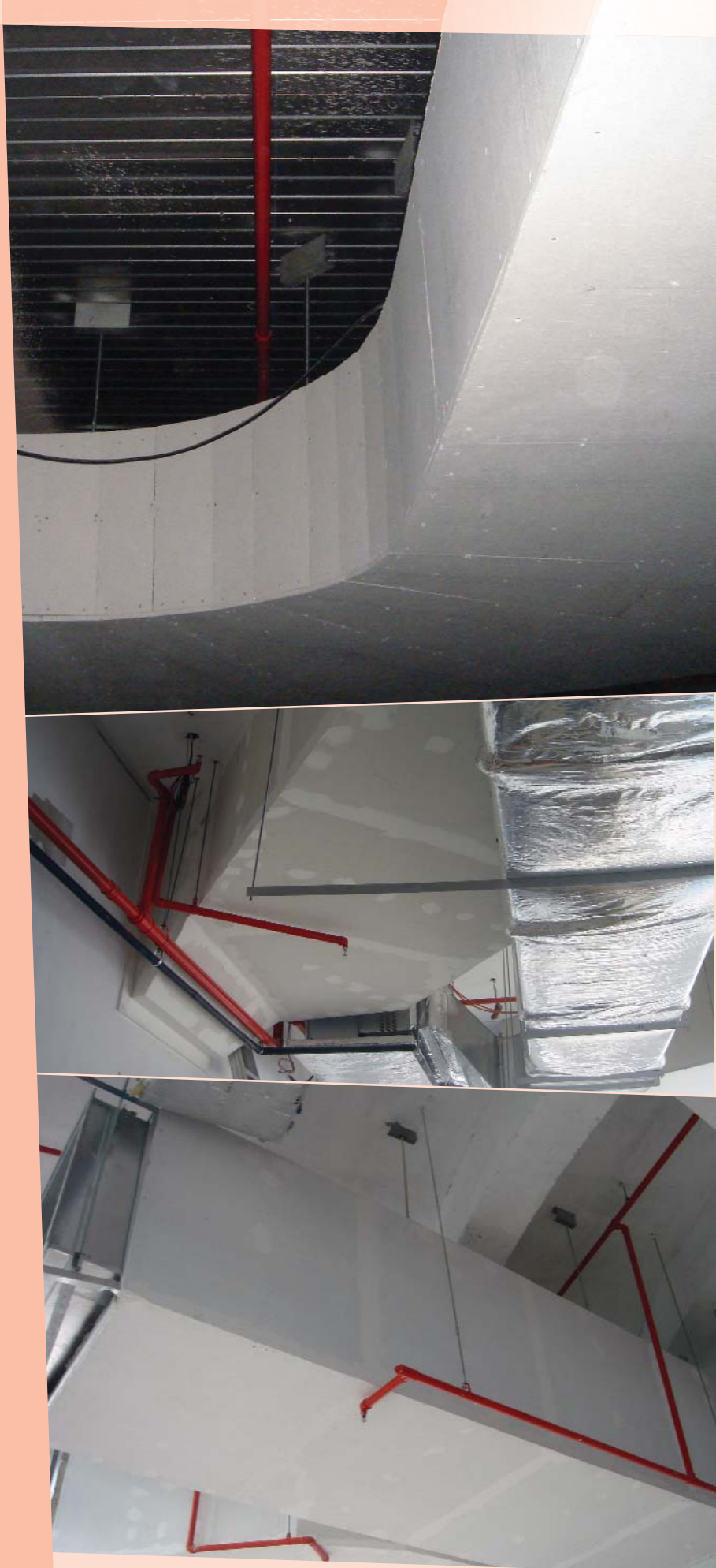
From top: SUPALUX® post cladding steel ducts in the solar panel plant of Renewal Energy Corporation, Park Hotel and ION Orchard, Singapore.
